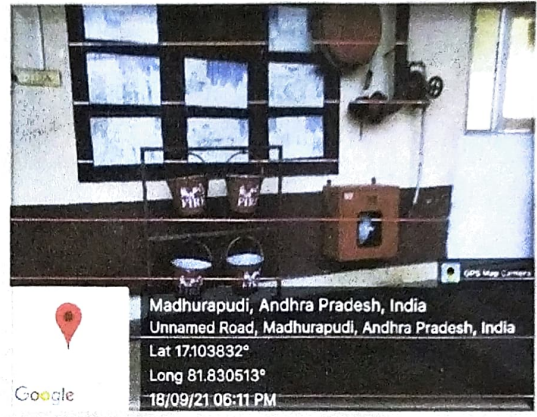
Fire safety pipe line
