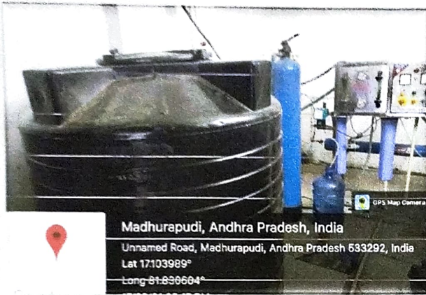
Reverse Osmosis Water Plant
